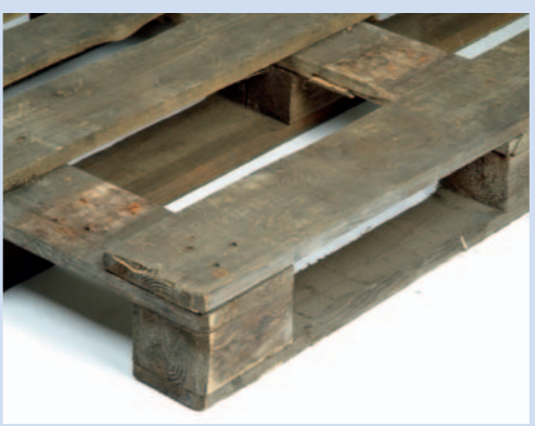
A board is missing.
